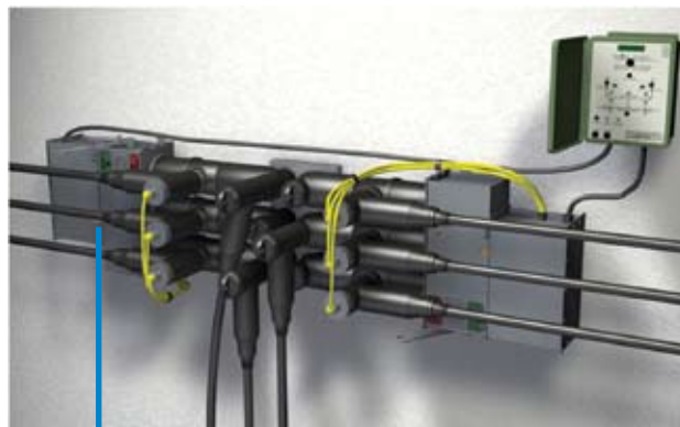
Wall Mounted Vault Installation
