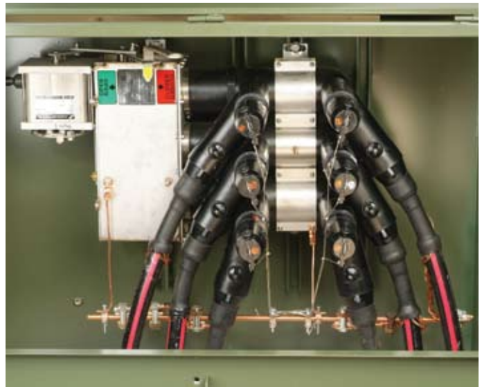
Motor Operated Switch
